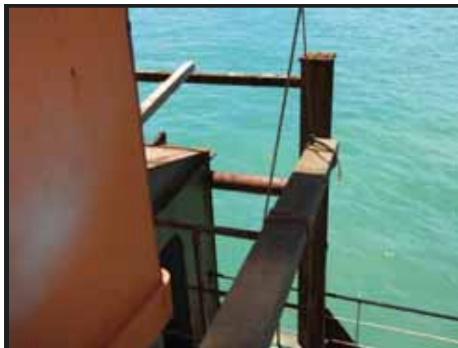
SAFETY? Some dodgy Dutch scaffolding aboard the Rotterdam
